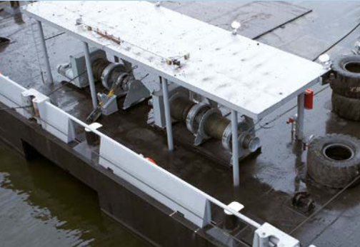
The crane's barge is also equipped with a number of winches used for warping the Floating Crane alongside sea-going vessels and for warping river vessels alongside the barge
